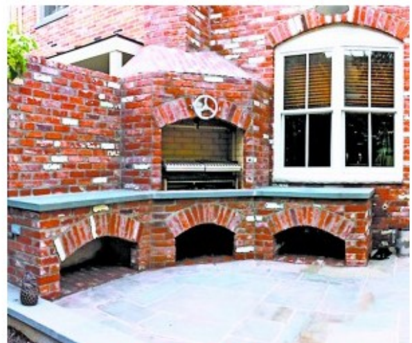
The Grillworks Architectural grill, installed with a new chimney on the back of this house using matching brick located by the architect, has the optional steel fire grates standing on the hearth.
